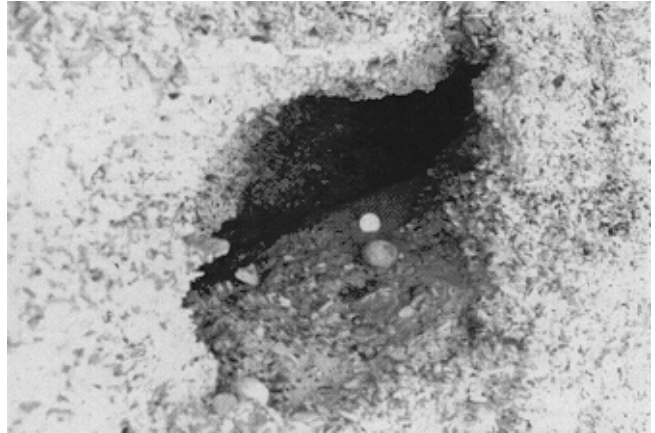
Figure 4-7. Piping and seepage in bank
