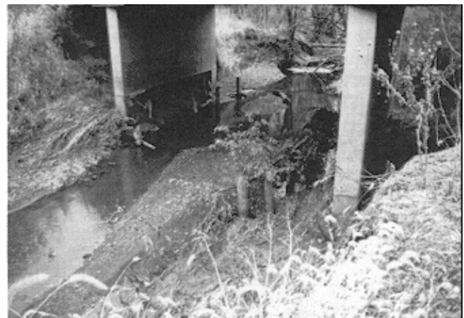
Figure 4-11. Exposed bridge piling
